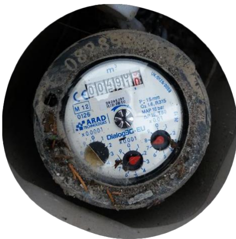
Left: You should ensure an internal stop tap is fitted on entry to the property.
